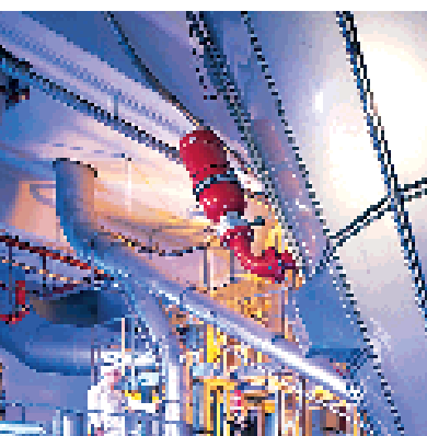
Suppressant safety system
