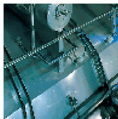
CIP nozzles for in-place cleaning
