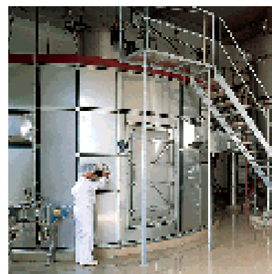
Removable insulation panels on drying chamber
